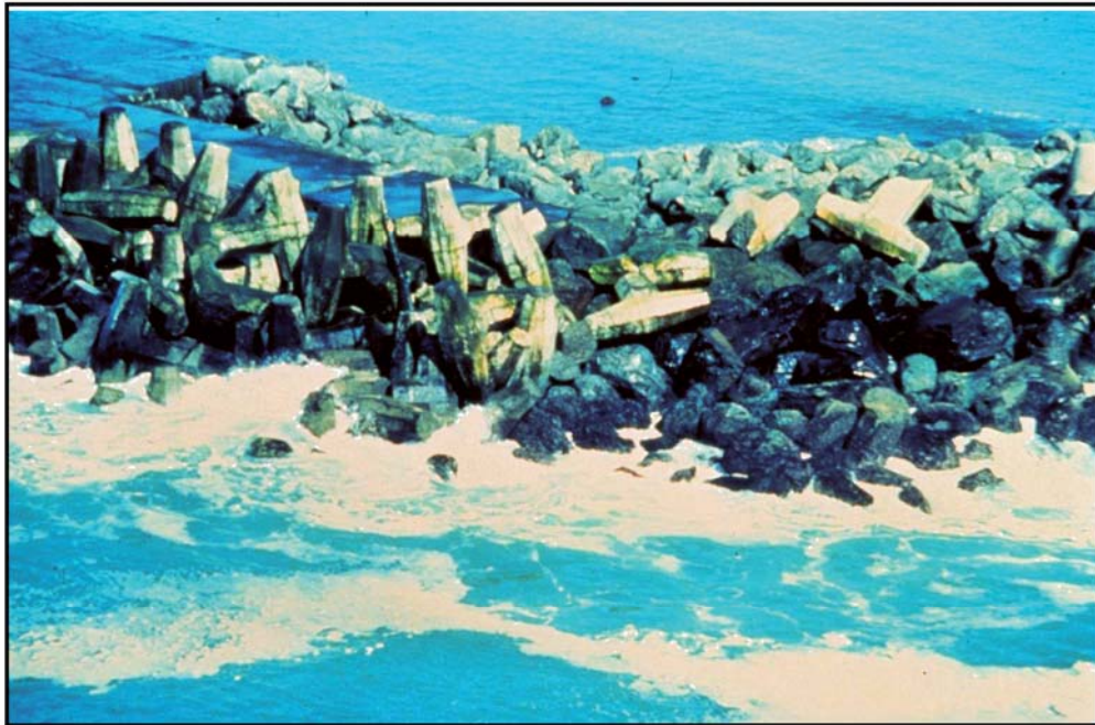
Breakage of armor units
